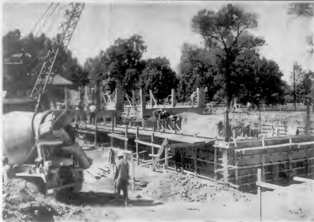
FROM THE GROUND UP—Construction is rapidly progressing on the new Humanities Building. The 1.3 million dollar structure, which is located between the Agriculture-Engineering and Old Science Buildings, is scheduled for completion by June 30, 1968.
